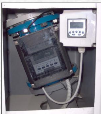
Flow meter of lime dosing German origin
